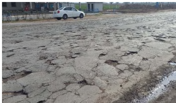
Pavement cracking in Termez district
