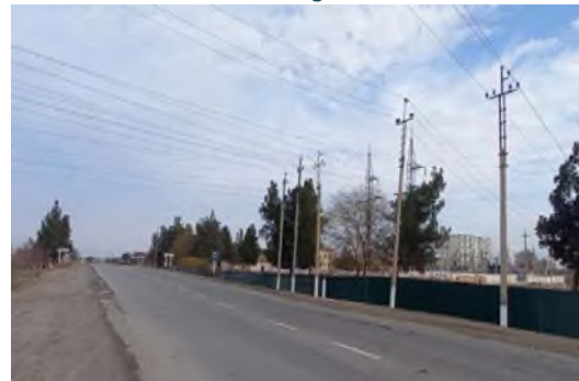
OHTL towers next to the road
