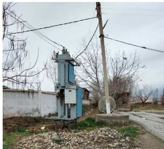
Transformer box in Kumkurgan district - 1530km
