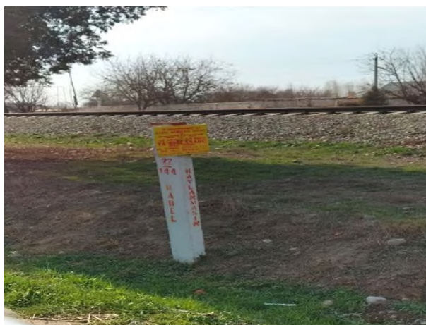
Communication cable in Kumkurgan district (15272km)
