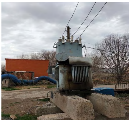
Transformer box in Kumkurgan district - 1535km
