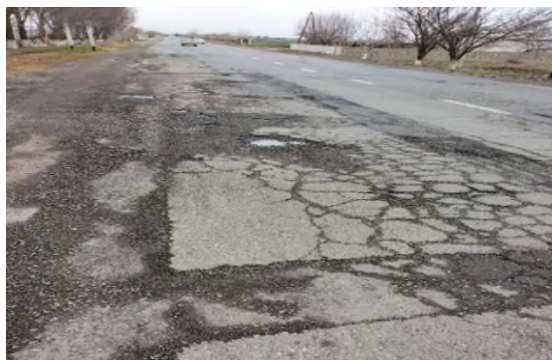
Pavement cracking and rutting in Kumkurgan district
