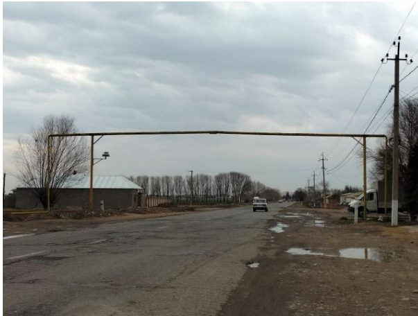
Gas pipeline over the road in Kumkurgan district (1531km)
