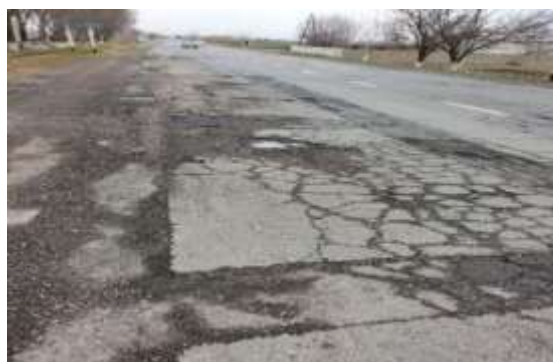
Pavement cracking and rutting in Kumkurgan district
