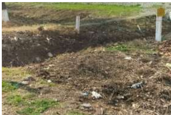
Existing underground cable in Termez district (1618km)
