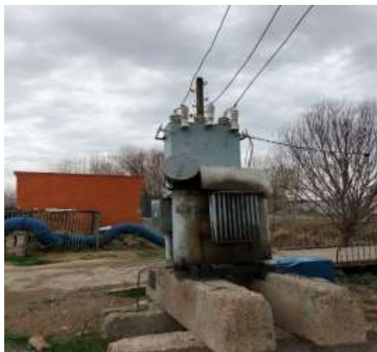
Transformer box in Kumkurgan district - 1535km
