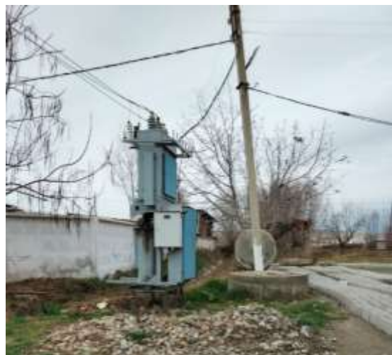
Transformer box in Kumkurgan district - 1530km
