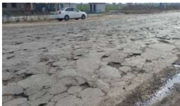
Pavement cracking in Termez district
